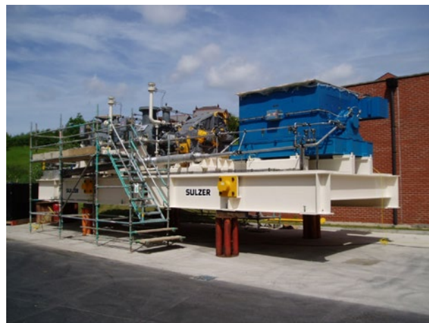
Figure 1: Natural gas compressor
