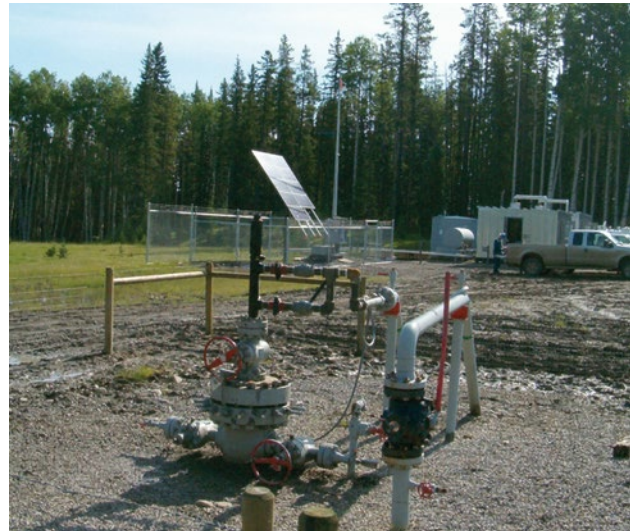
Figure 3: Solar chemical pump
