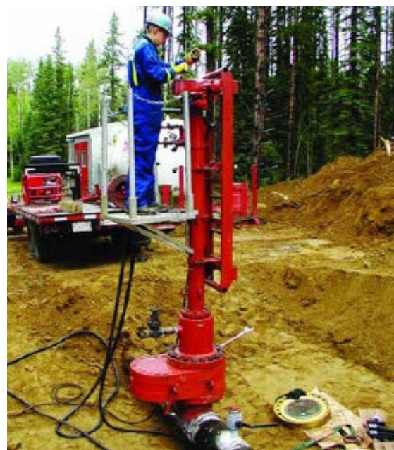
Certified Williamson Industries Technician performing a hot tap with a 760 Tapping Machine as part of a 123" Stopple application.
